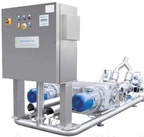
VIEW OF THE PUMP WITH DRIVE PROTECTIONS REMOVED
