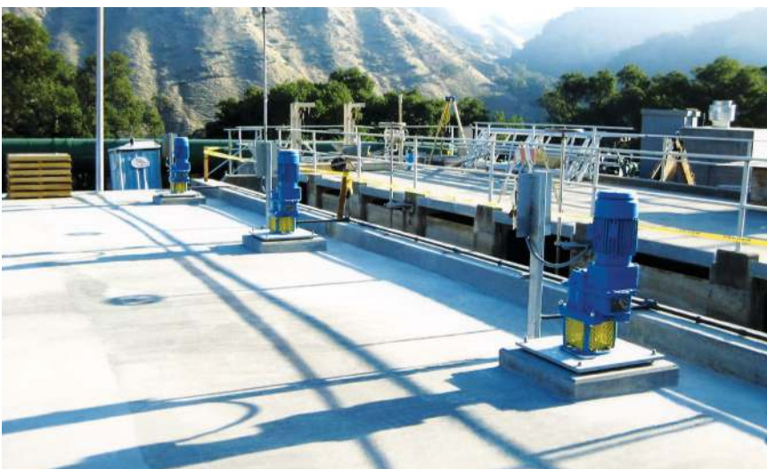
Installed Model 20 GTs at a wastewater treatment facility
